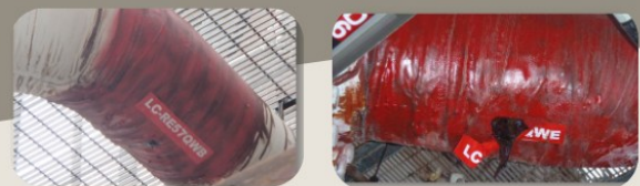
Figure 8: Composite repair failures
