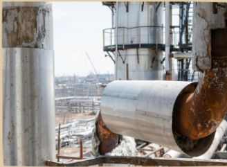
Figure 1: Corrosion of Insulated Pipe (Corrosion Under Insulation)
