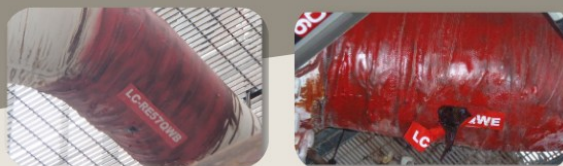
Figure 8: Composite repair failures
