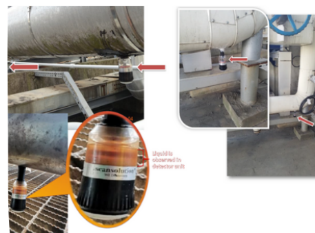
Figure 6: WI Discovery Leakage Detector with “photos” of installed locations.
